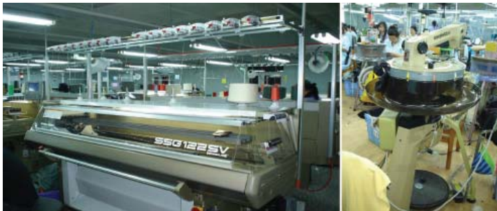
New Energy efficient equipment that has been installed
